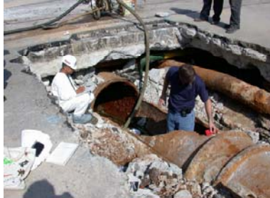
Broken 40-inch-diameter water main (© National Transportation Safety Board)
